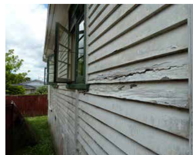
Severe rot in horizontal timber weatherboards.
