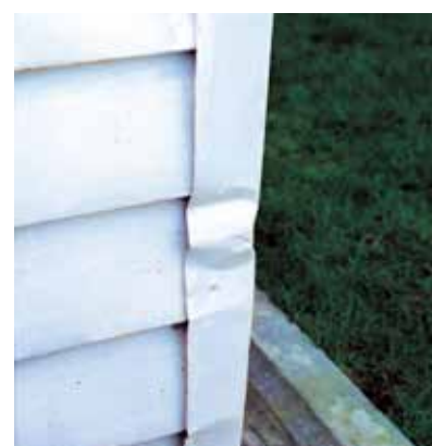
Impact damage to corner of metal cladding.
