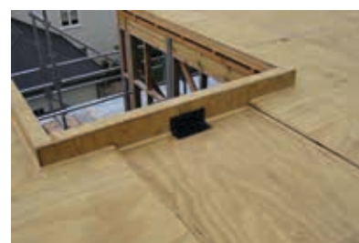
Incorrect use of fasteners can lead to deterioration of membrane and its adhesion or waterproofing.
