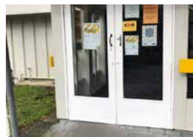
Timber door sill removed with paving built up to underside of door – potentially degrading bottom of door.
