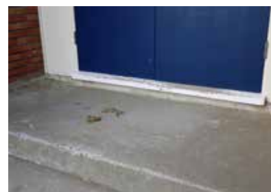
The door sill needs protection.
