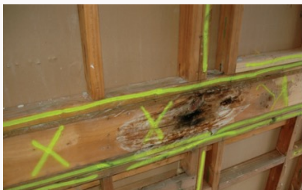
Evidence of a leak causing rot in timber framing.
