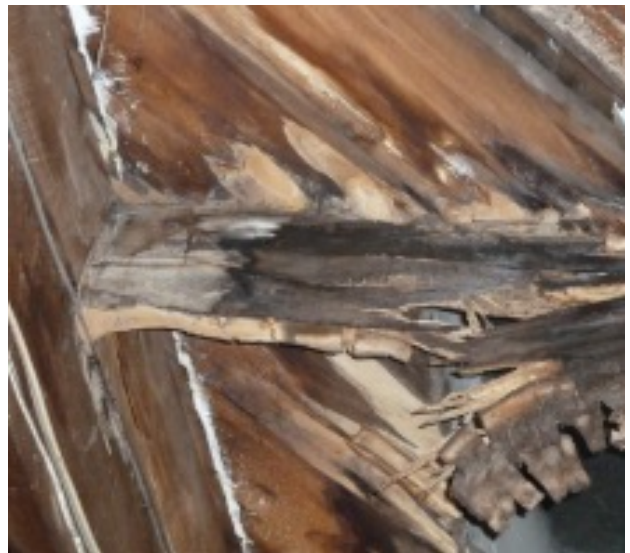
Damage from a large leak through the roof.
