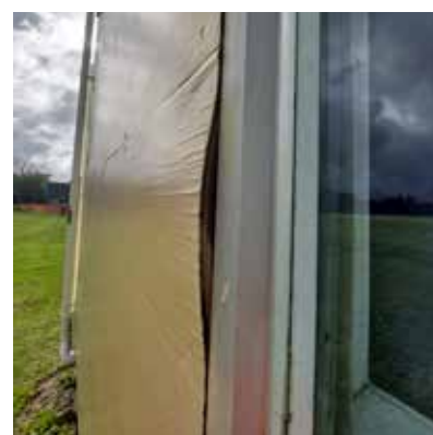
Cupping of plywood cladding.
