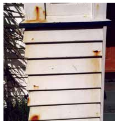
Rusty nail heads protruding through cladding.
