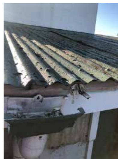
Roof and spouting requiring maintenance.
