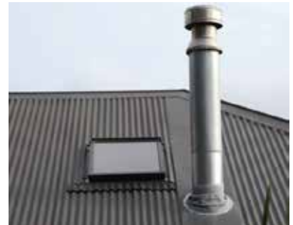
Flue stays not installed.
