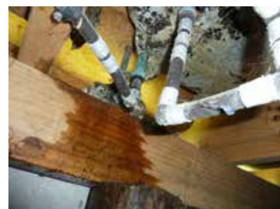
Leaking water pipe.
