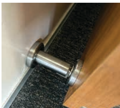
Door hold-open device.
