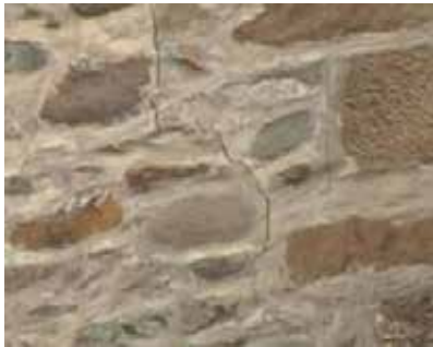
Cracking in stone wall.
