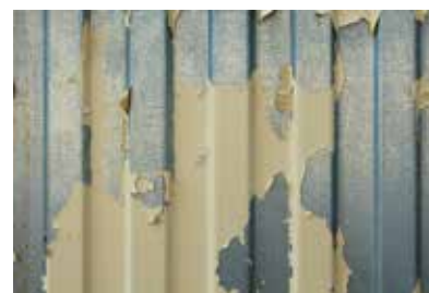
Paint peeling from metal cladding.
