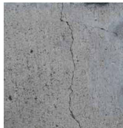
Hairline crack in concrete wall.
