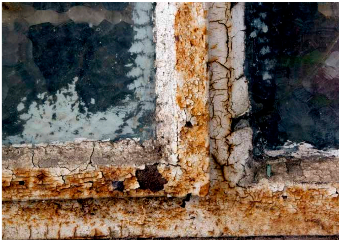
Severe corrosion on steel window frame.
