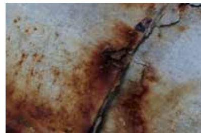
Severe rusting of metal surface.
