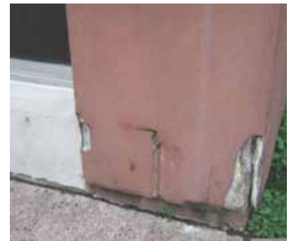
Cladding that is damaged and in contact with ground.
