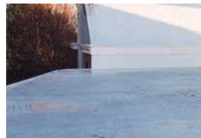
Insufficient fall to roof.
