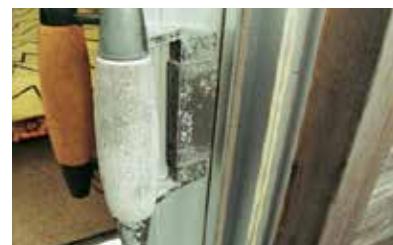
Surface deterioration on door hardware.
