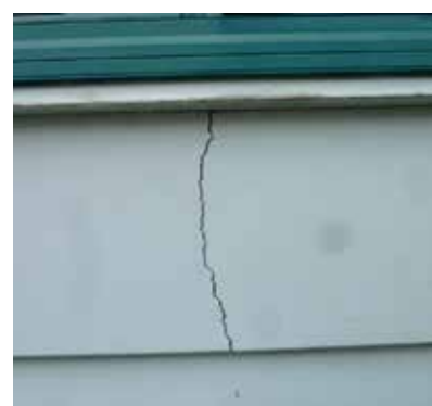
Cracking over full height of weatherboard – consider urgent repair.
