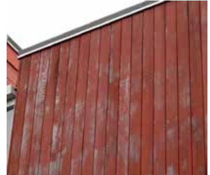
Plywood showing signs of needing to be painted.
