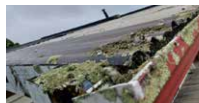
Lichen on gutter.
