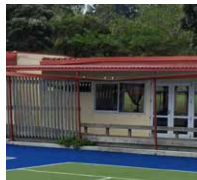
Gutter requiring urgent repair.
