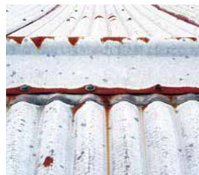
Red rust on galvanised roofing.
