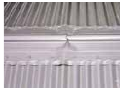
Ridge flashing buckling due to thermal expansion and contraction.
