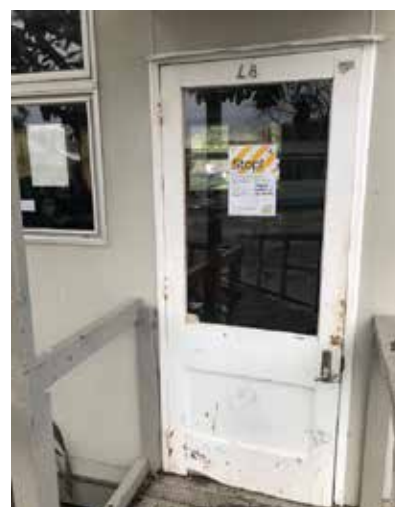
Broken handle to exterior door.
