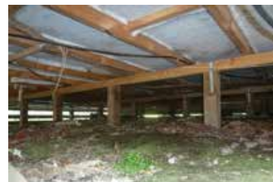
Lack of bracing to piles.
