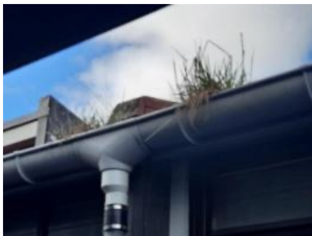
Vegetation blocking the spouting causes water to overflow and make the accessway below slippery.
