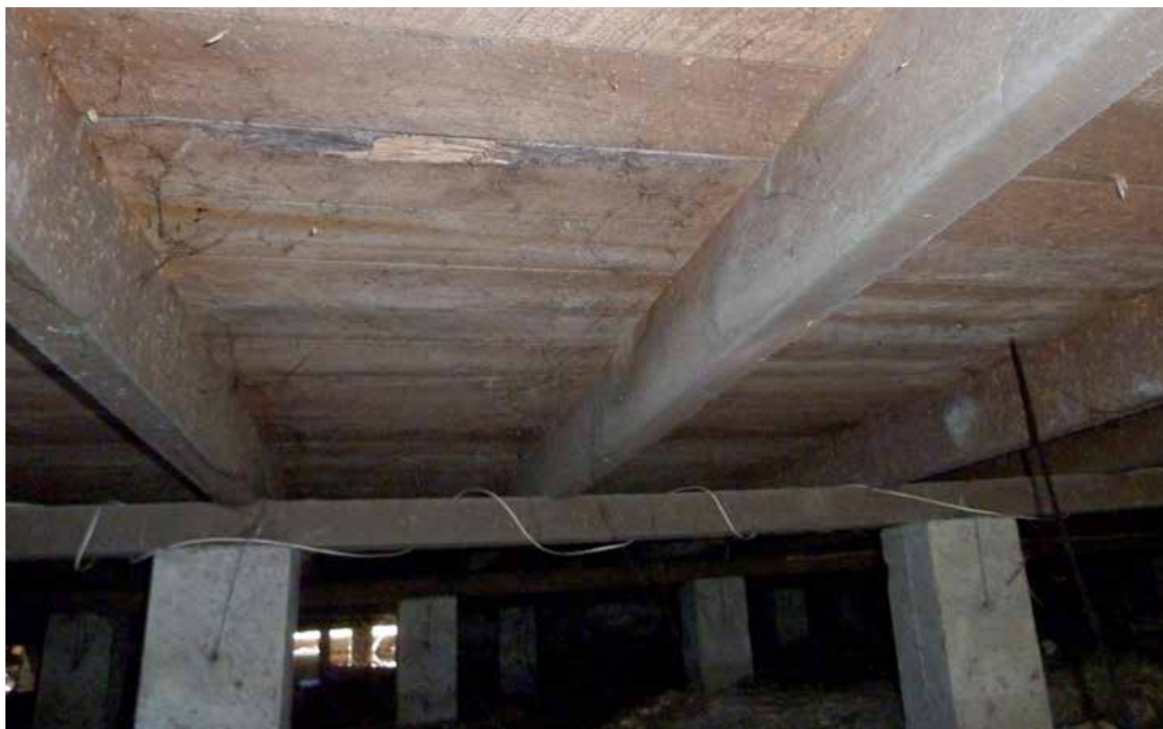
No subfloor insulation.
