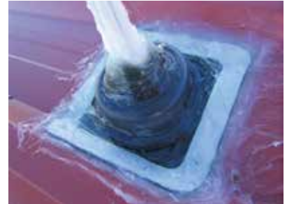
Roof penetration inadequately sealed.
