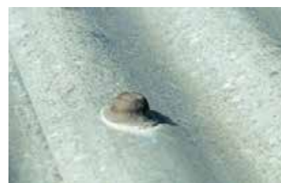
White rust around nail head.
