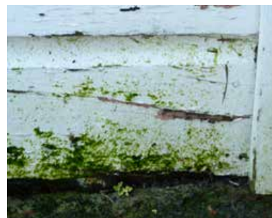
Degrading weatherboards at base of exterior wall.
