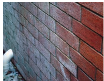
Efflorescence on brick veneer.
