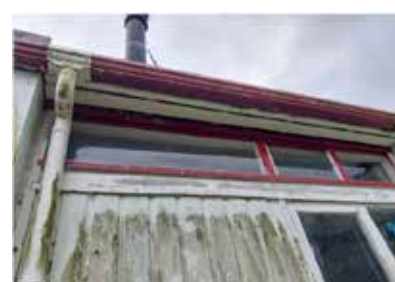
Spouting requiring urgent repair.
