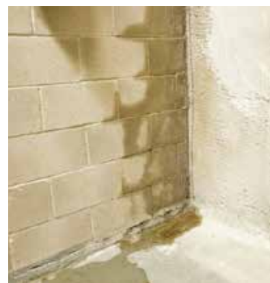
Basement wall showing signs of water penetration.
