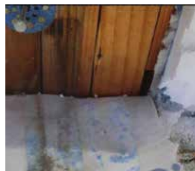
Impact damage causing failure of cladding system.
