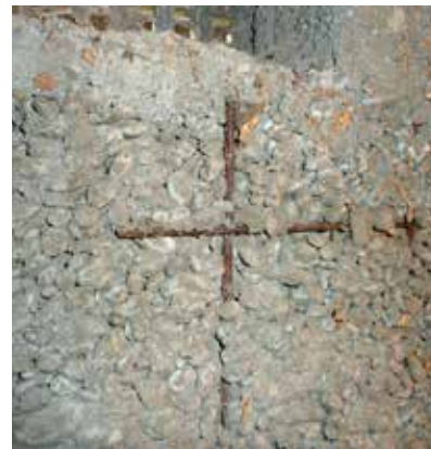
Inadequate installation of reinforcing causing rusting – consider urgent repair.
