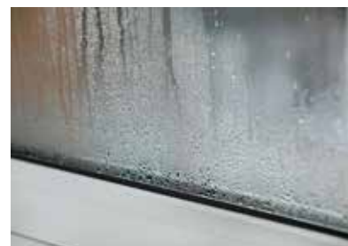
Moisture in double-glazed unit.
