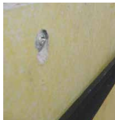
Signs of coating failure at panel fixing.
