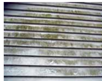
Moss, mould and lichen growth evident on timber cladding.
