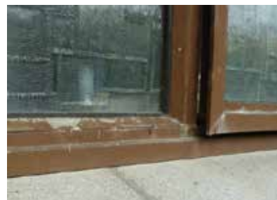
Coating failure on aluminium window.
