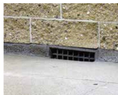
Subfloor ventilation is limited by concrete paving.
