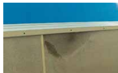
Soffit damage due to leaking gutter.
