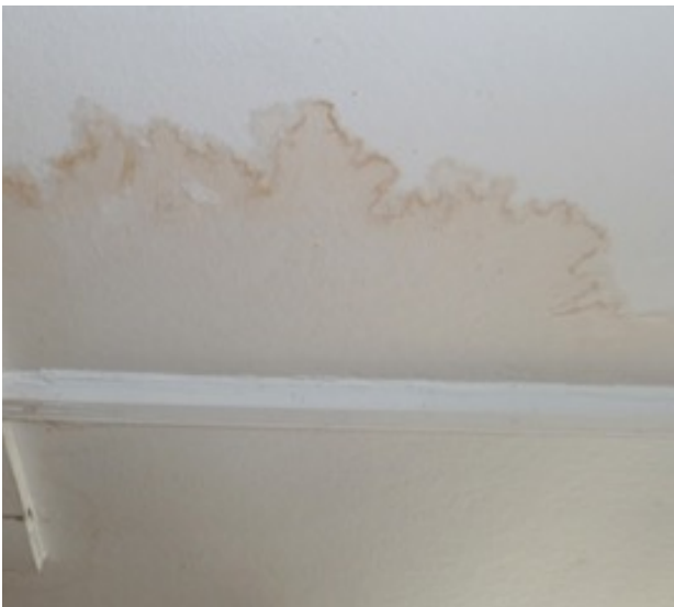
Evidence of a small leak in the ceiling or the start of a larger leak.
