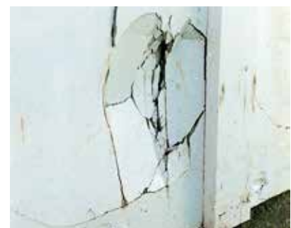
Impact damage to sheet - consider urgent repair.
