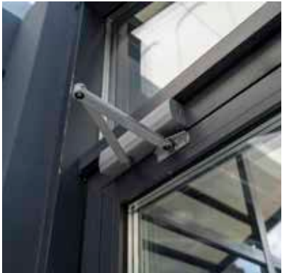
Self-closing door hardware to exterior door.
