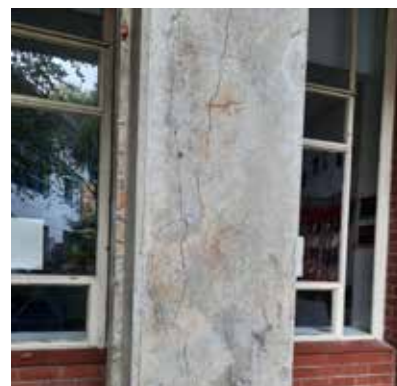
Serious spalling and cracking of concrete wall – consider urgent repair.
