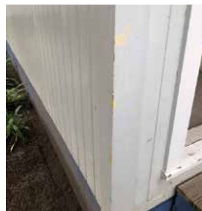
Dirt splashed up onto baseboards.
