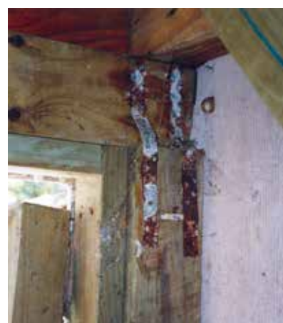
Rusted connections to jack stud framing.
