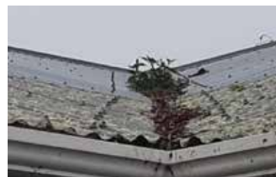
Debris on roofing.
