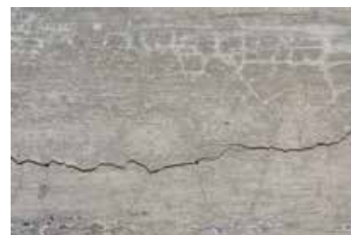
Cracked concrete wall in need of repair.
