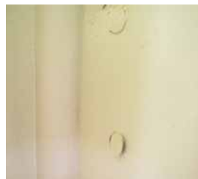
Nails popping through cladding.
