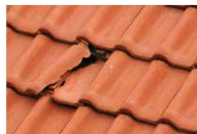
Cracked clay tile.
