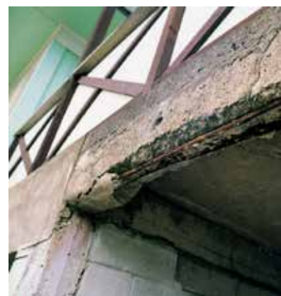
Serious corrosion of reinforcing causing cracking of concrete – consider urgent repair.
