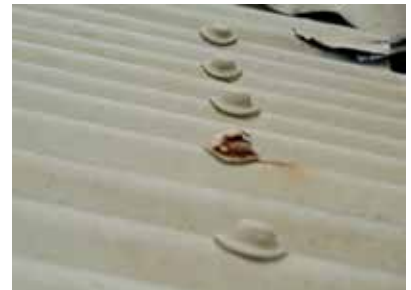
Corrosion of fixings.
