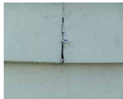
Crack appearing in weatherboard cladding.
