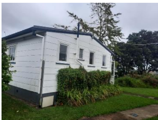
Plants affecting the performance of the cladding.
