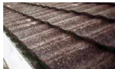
Loss of stone chip coating.
