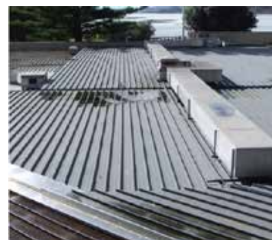
Insufficient fall causing ponding on roof.
