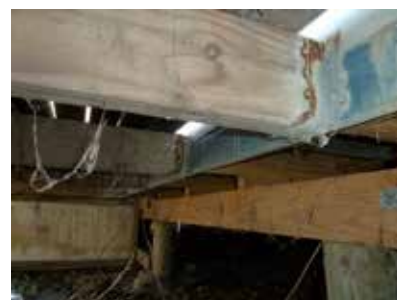
Rusting joist hangers.
