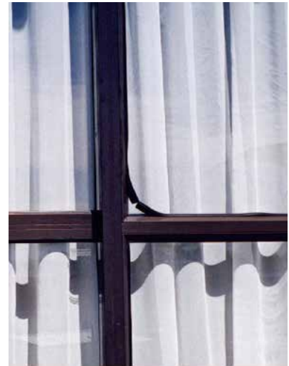
Failed rubber seals.
