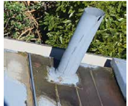
Corrosion of roof around penetration.
