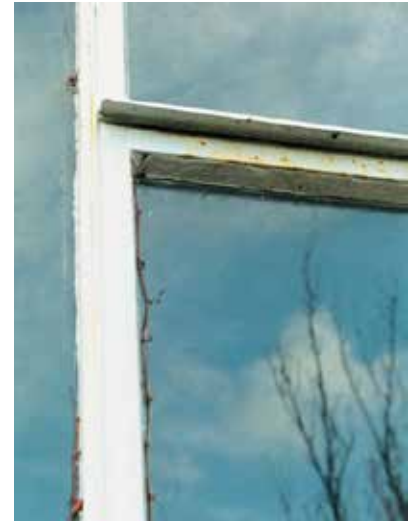
Signs of surface rust appearing on steel window frame.
