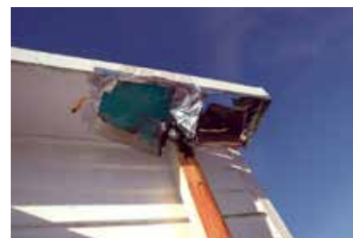
Joint failure in gutter.
