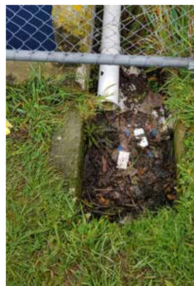
Blocked sump causing dampness around exterior retaining wall.
