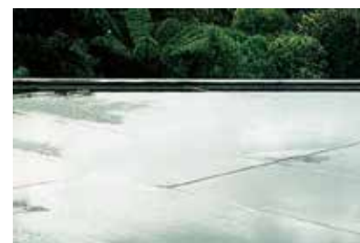
Water ponding on membrane roof.
