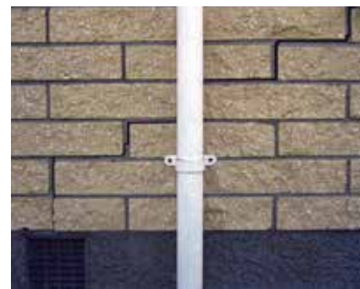
Cracks in veneer consistent with building movement or settlement.
