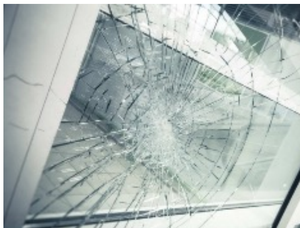
Impact damage to a glass panel.
