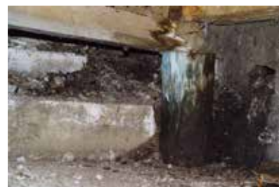
Piles showing signs of timber decay.
