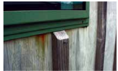
Plywood with no paint or stain protection.
