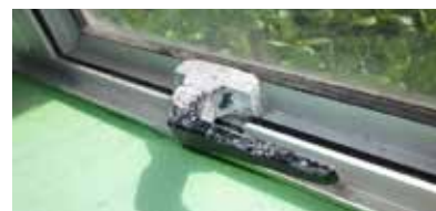
Surface deterioration on window hardware.
