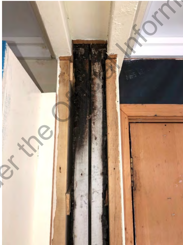
Figure 3: Fire damage to structural column at Block B
