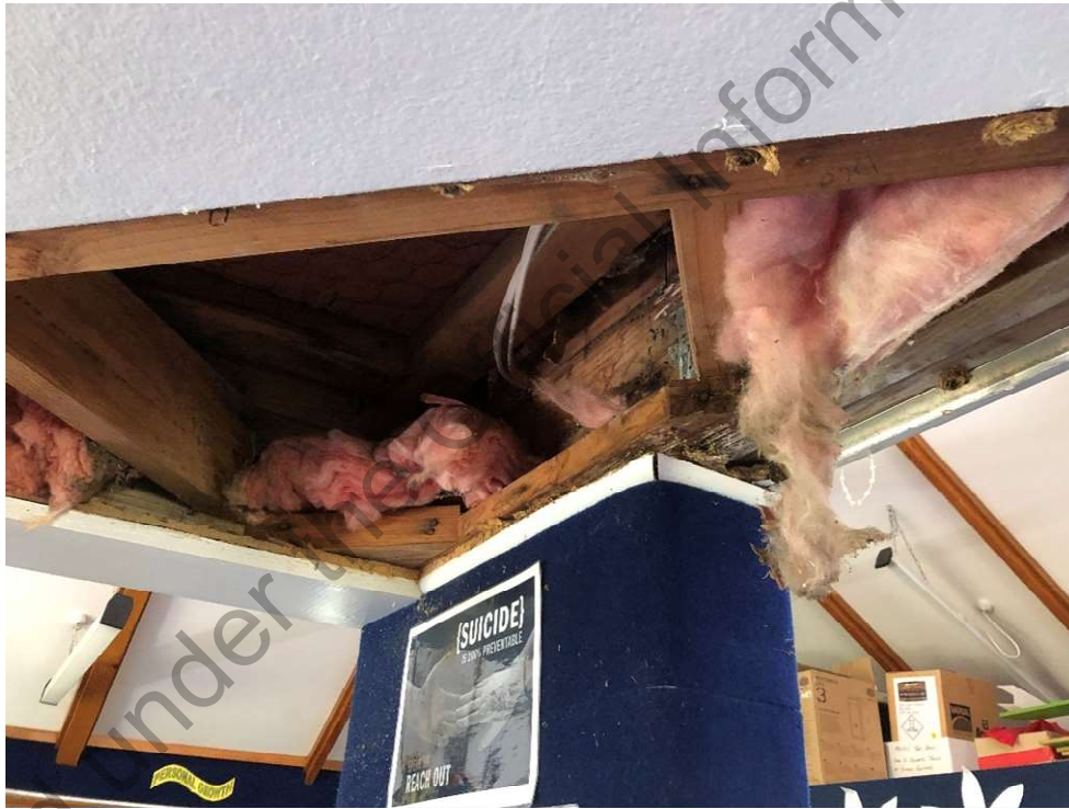
Figure 5: Evidence of decaying roof structure at Library
