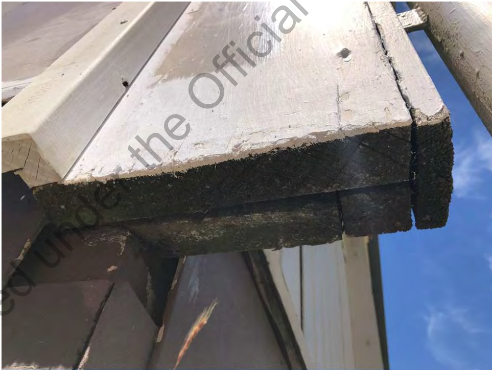
Figure 2: Example of portal leg with decayed timber and minimal bearing at Block B
