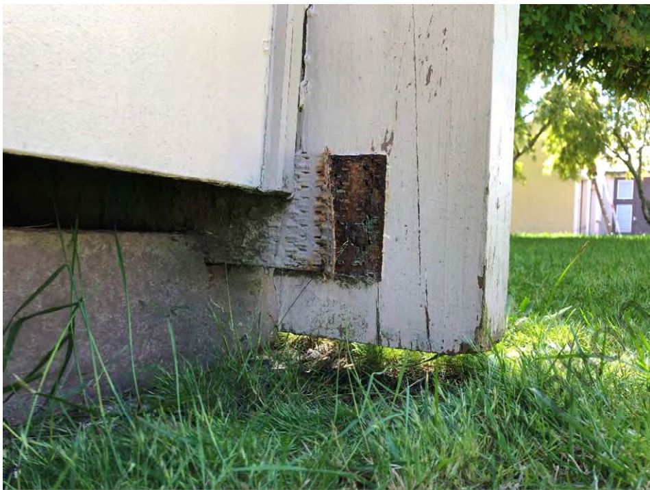
Figure 1: Example of portal leg near ground with gang nail plate separation at Block R
